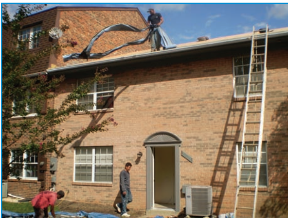
John Darvish Construction employees work on the roofs of two townhouses for Good Shepherd Housing & Family Services.
